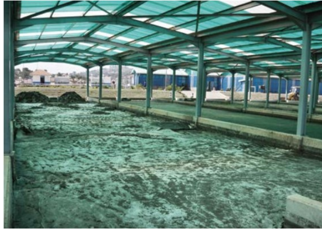
Drying beds at Lubigi Wastewater and Faecal Sludge Treatment Plant in Kampala, Uganda
